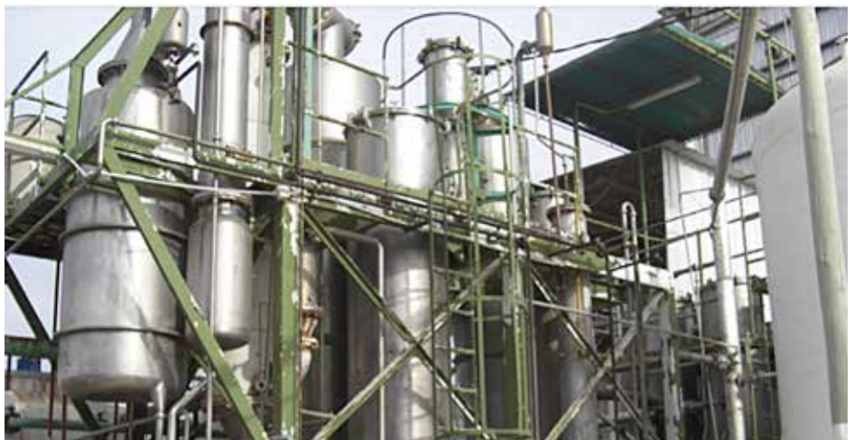
Whey processing facility in Argentina.
